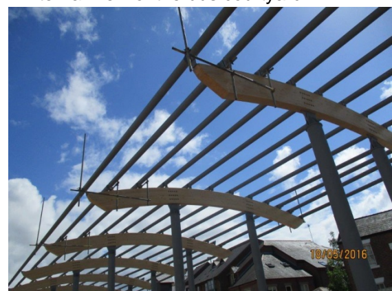
Edge Protection being put in place prior to commencing the roofing works.
